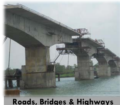
Roads, Bridges & Highways Construction of bridges, elevated metro, concrete pavements for airports
