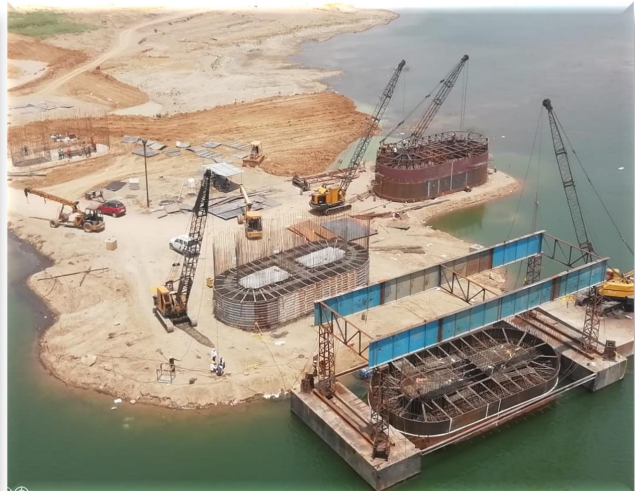
Dhaulpur Project Executed Caissons for Double - D well foundation in a perennial river Condition
