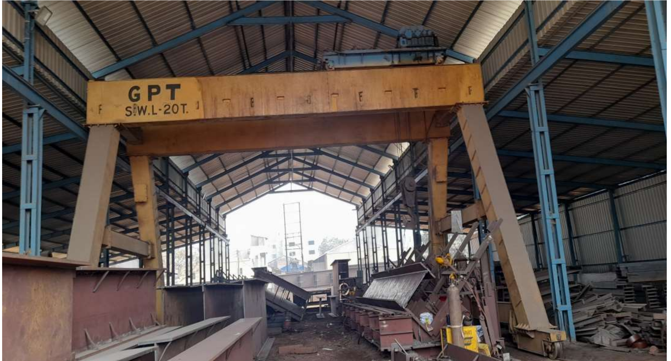
GANTRY CRANE -20T
