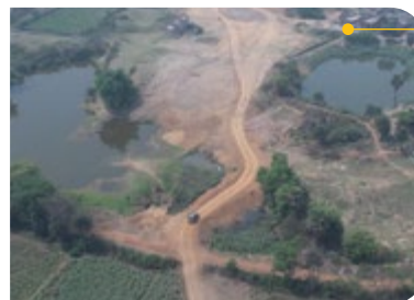
Building a 4-lane Raniganj Bypass on NH-60 in Paschim Bardhaman, West Bengal.
